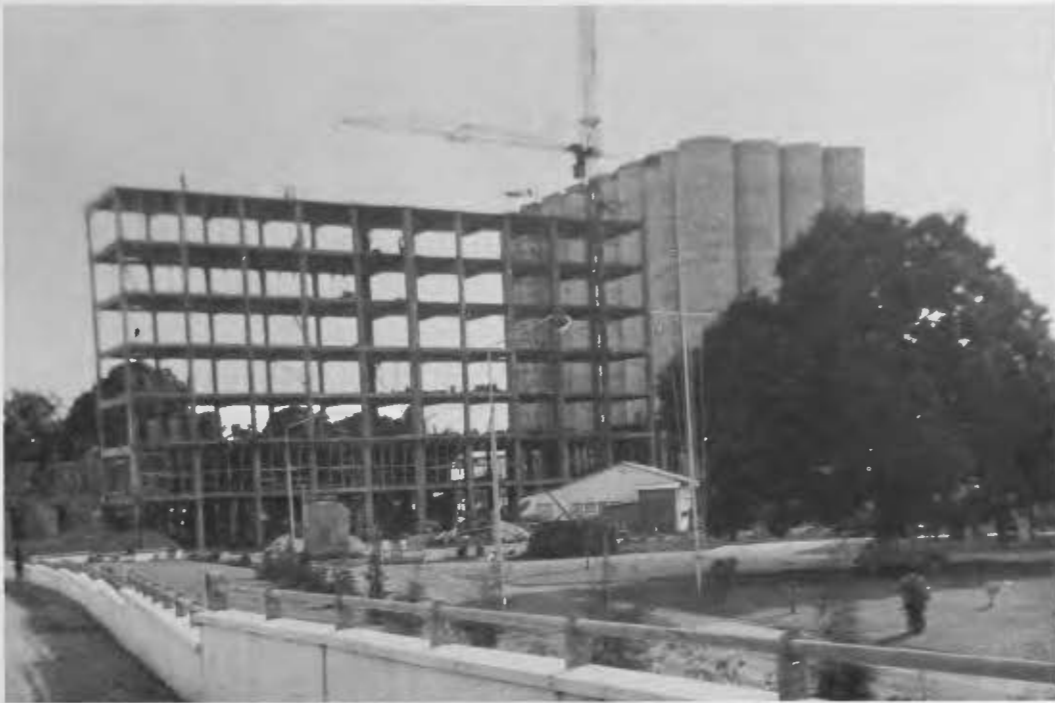
Figure 12.--Flour mill at Abidjan while under construction. While now obligated to grind only franc-zone wheat, the mill offers a potential future market for U. S. wheat. The Ivory Coast grows no wheat.
